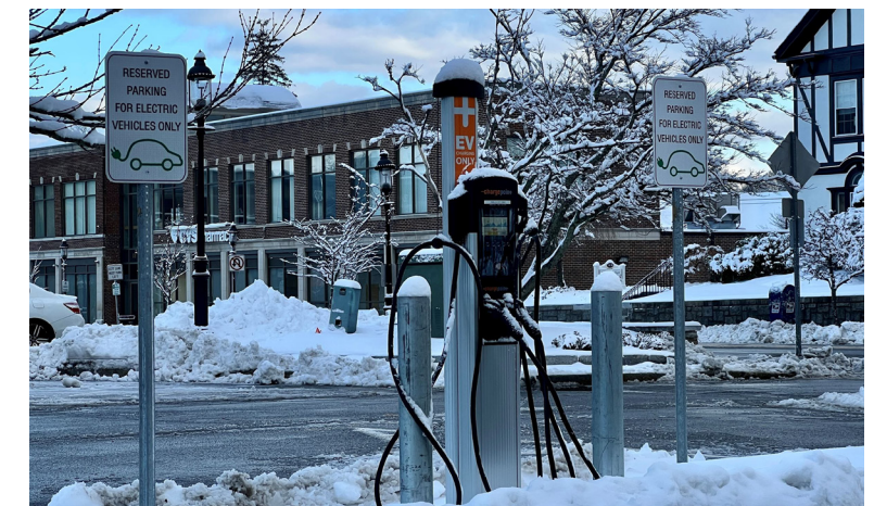
Electric Vehicle Charging Station at 89 Main Street.
