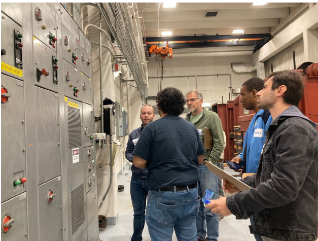
UMass Amherst's Industrial Assessment Center faculty and students visit Andover's Water Treatment Plant for a comprehensive tour and energy assessment. Photo by Joyce Losick-Yang.
